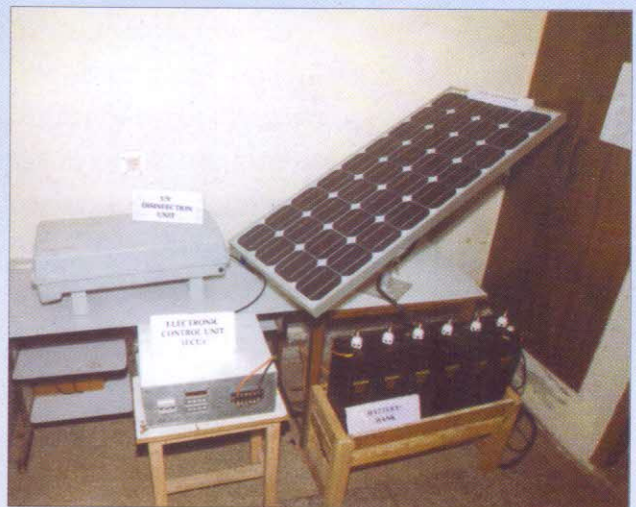
Solar PV Power Drinking Water UV Disinfection Plant
