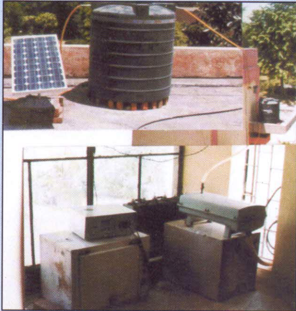
Solar Power Drinking water UV Disinfection Plant installed at Haiderpur Water Works, Delhi Jal Board, New Delhi.
